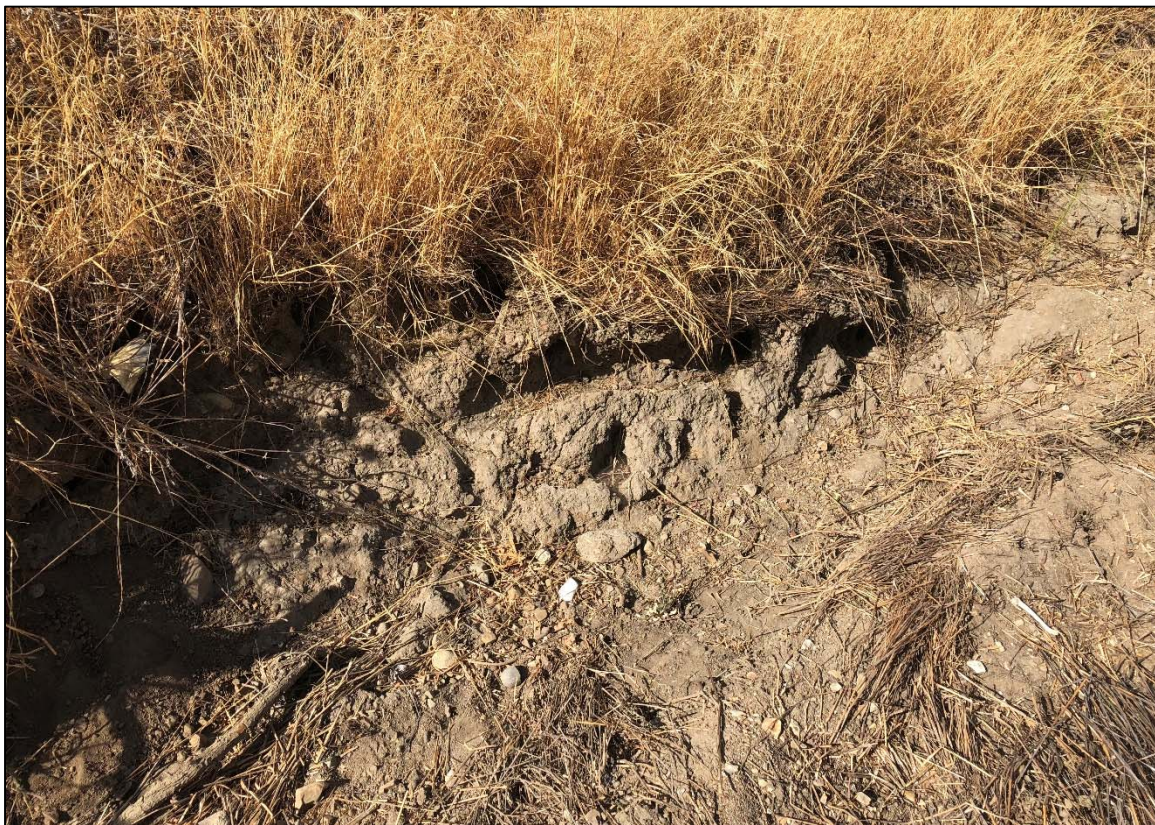
Erosion near the culvert and concrete ditch that directs stormwater run-off onto the north corner of the property.
