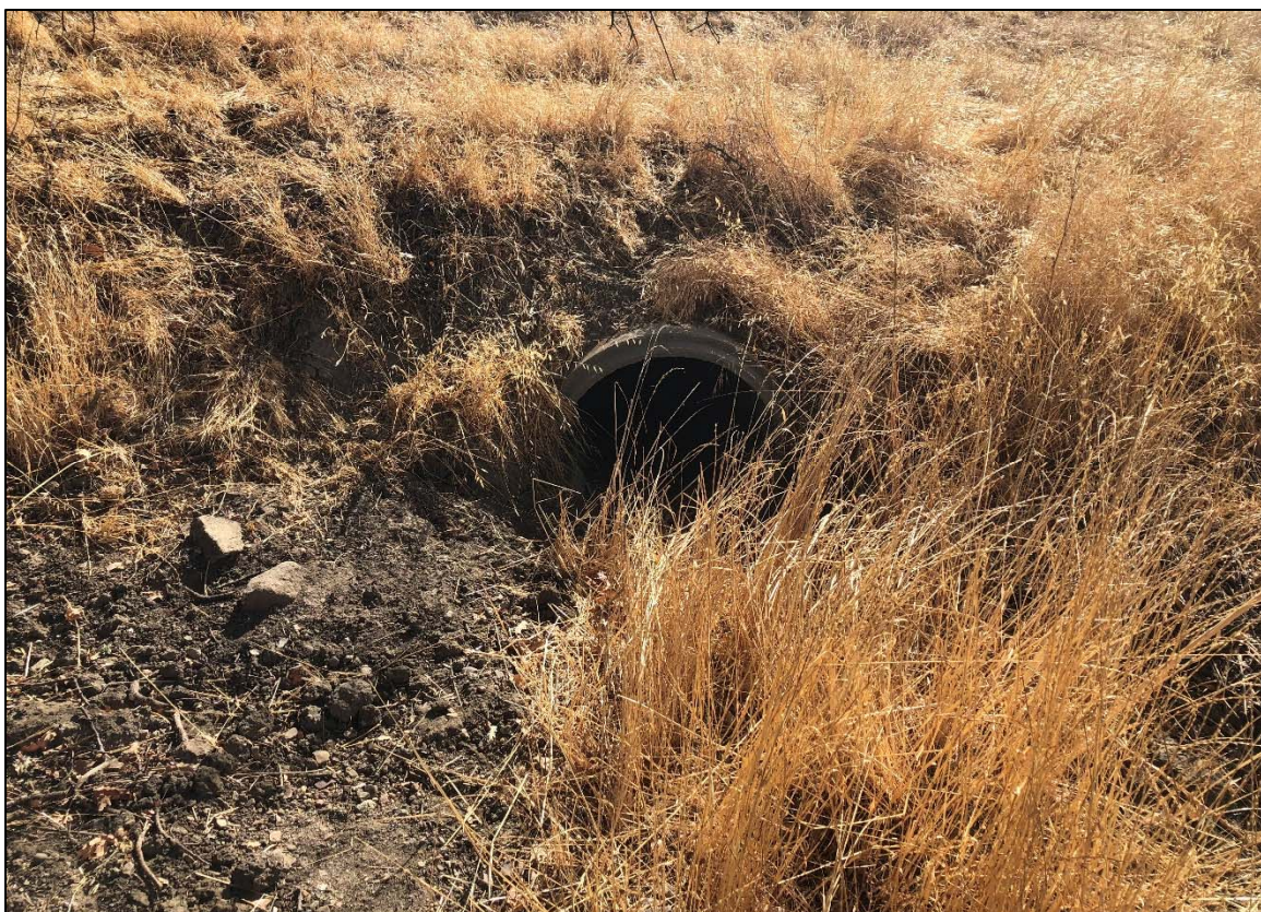
Culvert directing stormwater run-off from Highway 101 onto the property.
